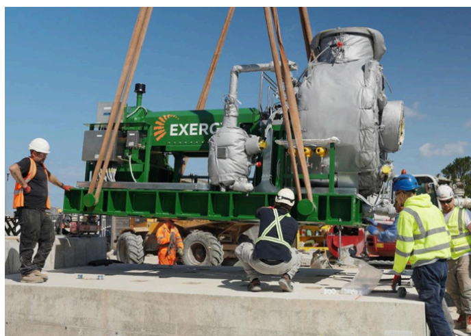
Radial Outflow Turbine onsite construction at United Downs in Cornwall uses a binary plant to generate electricity and support lithium-extraction operations from deep geothermal fluids.
